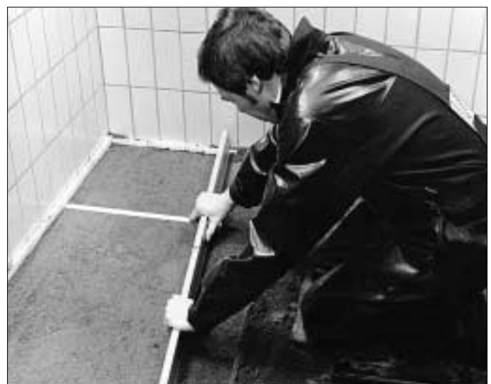
4. Position the guides at intervals of 2–3 metres, or at any other distance that is appropriate with respect to the area to be tiled. The mortar should be levelled at the right height according to the guides.
