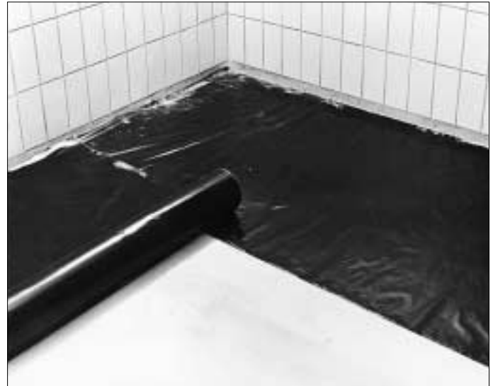
2. A 0.1 mm plastic sheet should be unrolled on the sub-floor. A soft brush should be used to smooth out the sheet and remove any air bubbles. Roll out each sheet so that it overlaps the preceding one.
