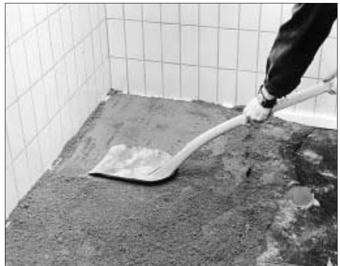
3. Spread out the mortar and compact it carefully. Do not spread out more mortar than is needed for 4–5 courses of tiles at one time.
