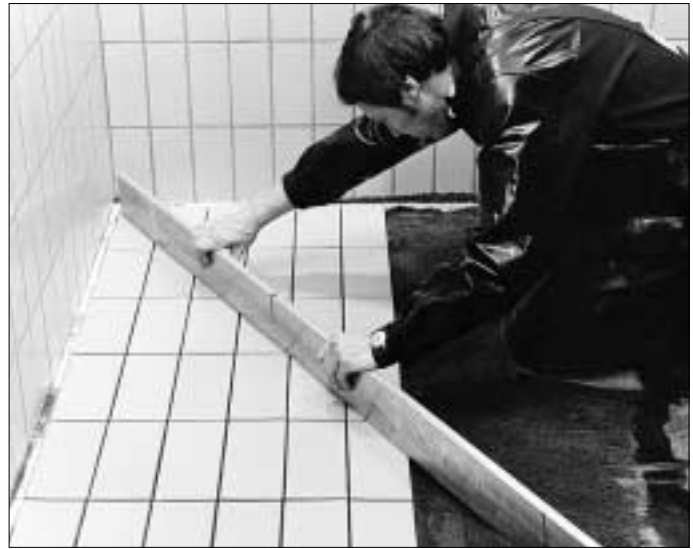
8. The evenness of the surface of each newly laid section should be carefully checked with a gauge float and adjusted if necessary.
