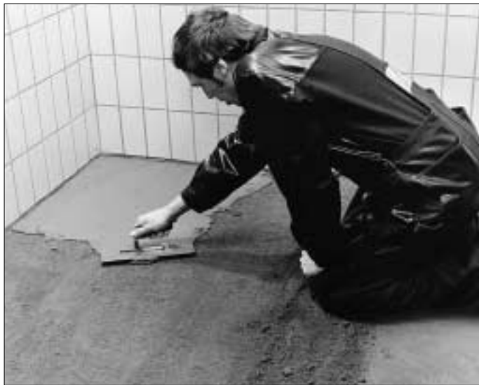
5. A fluid cement slurry (cement and water) should be spread over the bedding mortar.
