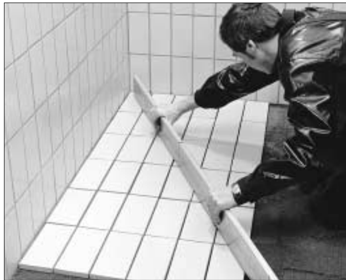
8. The evenness of the surface of each newly laid section should be carefully checked with a gauge float and adjusted if necessary.
