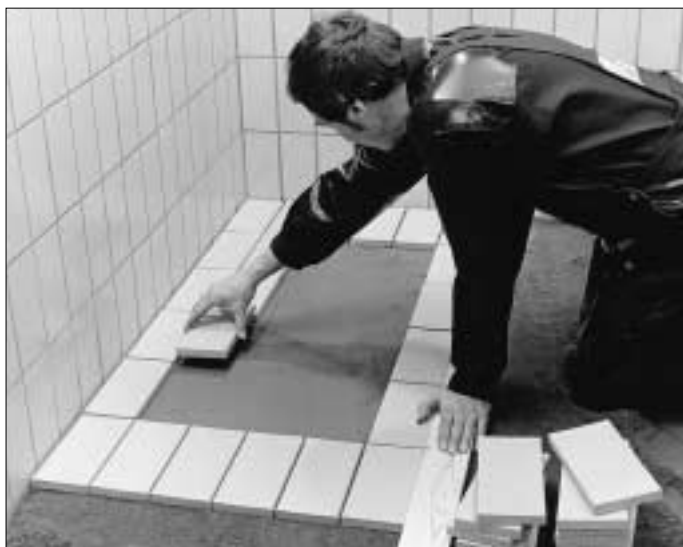
6. When the surplus water has been absorbed by the mortar and the slurry has taken on a matt appearance, the tiles should be laid out according to the markings on the gauge float.
